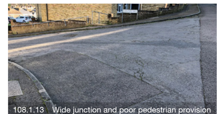
108.1.12 Lack of traffic calming †
