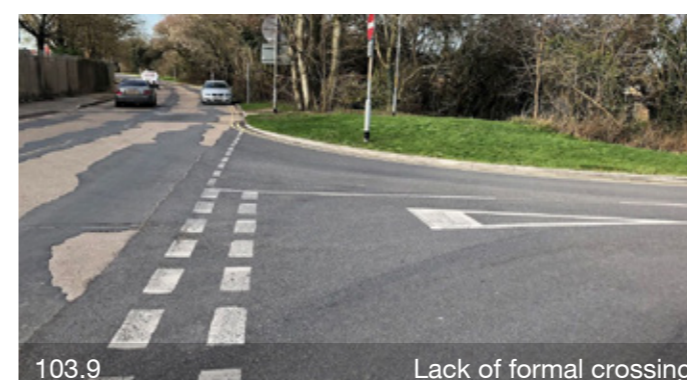
103.8 Wide junction and poor pedestrian provision
