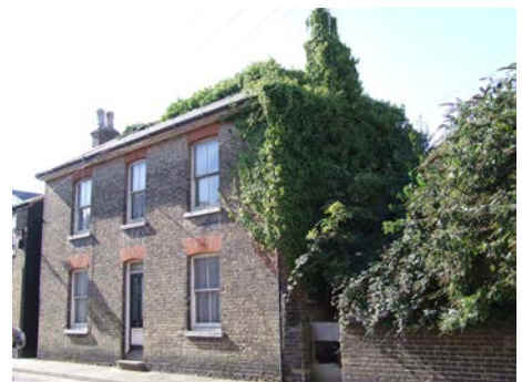
37 Nelson Street, in a state of disrepair at the time of the appraisal
